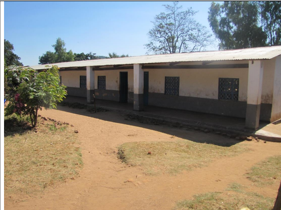
One of the school blocks at Kaduku Primary School that had been blown off and later received CDF funding to re-roof the structure in Rumphi west Constituency
